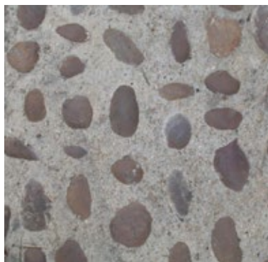
Incorrect river pebble paving
