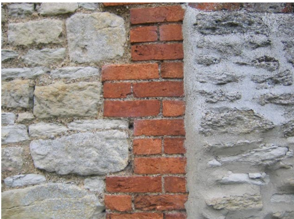
Examples of good and bad pointing
