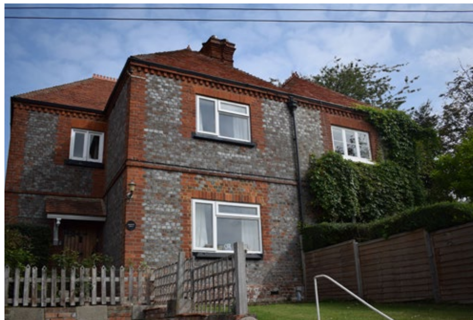
Fig 28. Dharwar Villa, which has had its original casement windows replaced
