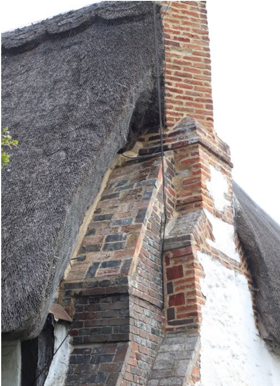
Fig 18. A variety of building materials and techniques on the road facing gable end of The Thatch
