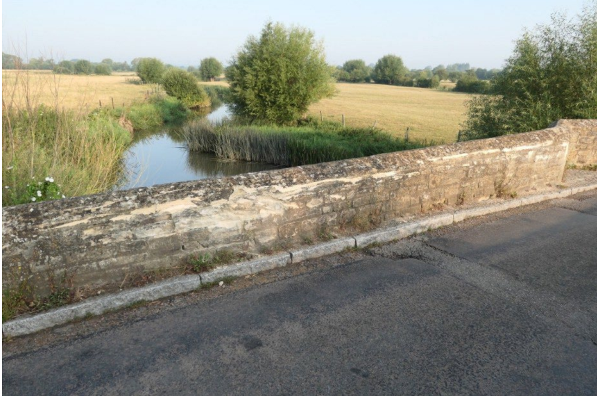
Fig. A7.1 Cumulative collision damage caused to Ickford Bridge, 12/08/2020
