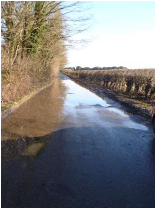
Fig.24: Flooding on Pyrton Lane (February 2014)
