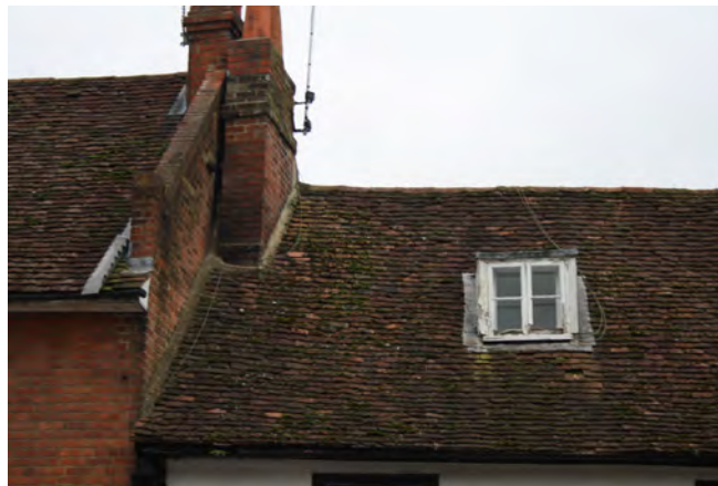
Timber windows in need of repair and moss growth to roof tiles
