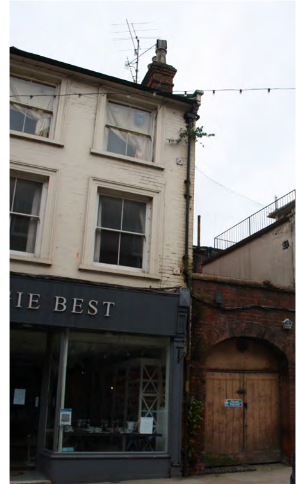
Damaged drainage goods and foliage growth
