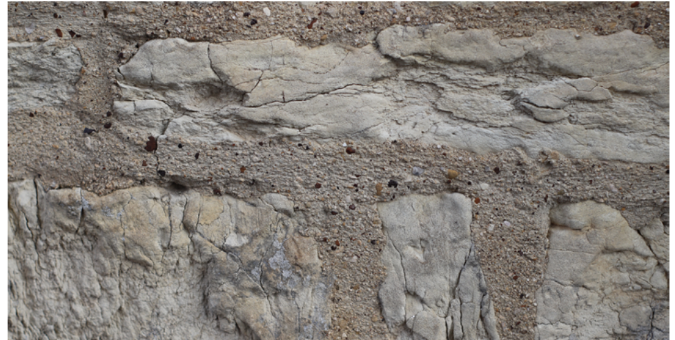
Fig 15. Chalk clunch wall and lime mortar.
