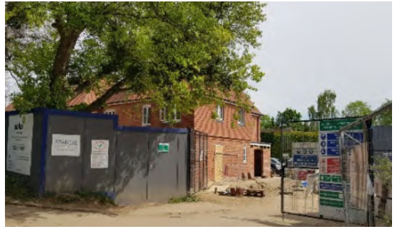
Figure 116: There are number of properties under construction, such as these in Mill Road, which replaced Sydney Harrison House. The new flats and houses being constructed have been designed to follow the dominant building line
